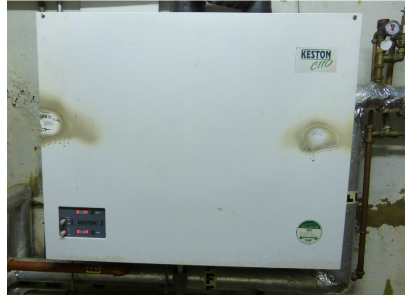
Boiler showing two failure points where the casing melted from escape of hot combustion gases from Heat Exchanger.
